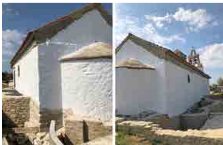
Fig. 26. Inadequate conservation treatment of external faces of the walls on the present-day Orthodox parish church of Sts Joachim and Anna at Bribir (photo: A. Milošević)
