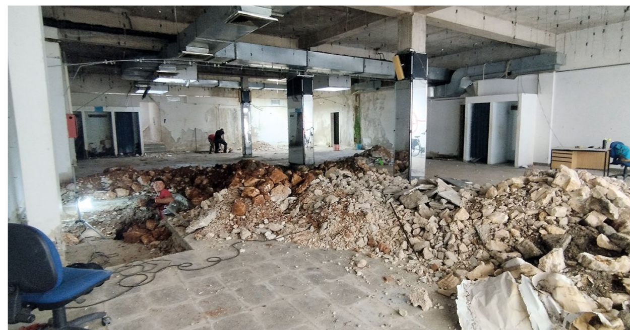
Stražnja zgrada unutar koje su kopane prve četiri sonde (foto: F. Jurković Pešić) The rear building inside which the first four trial trenches were dug (photo: F. Jurković Pešić)
