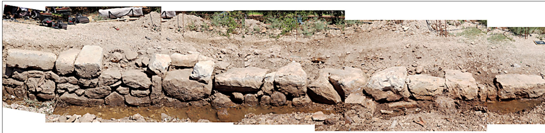
Snimka podzida obale (izradila: A. Matura) Image of the retaining wall (made by A. Matura)
