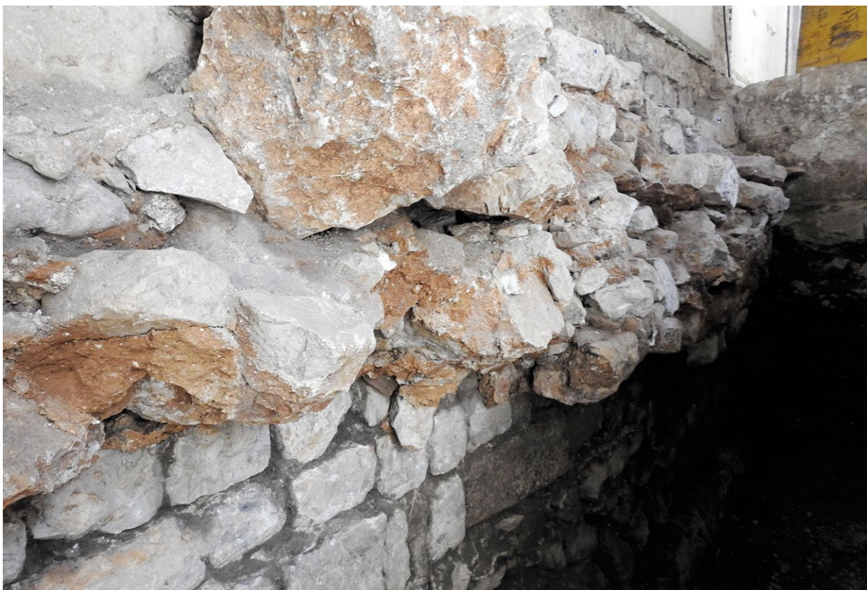
Detail temeljne stope s kasnijim popravcima (foto: F. Jurković Pešić) Detail of the footing with later repairs (photo: F. Jurković Pešić)
