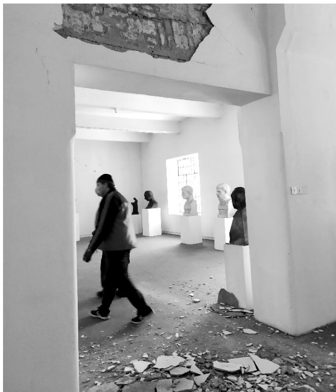
Figure 4. Big cracks on the walls and ceilings in the interior (Source: Photographic Collection of the Glyptotheque)
